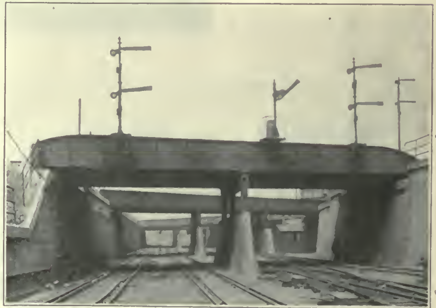
FIG. 268. BRIDGES. Through plate-girder bridges over the Chicago & Western Indiana Railroad at 16th Street, separating crossings of the Lake Shore & Michigan Southern Railway, the Chicago, Rock Island & Pacific Railway and the St. Charles Air Line.
